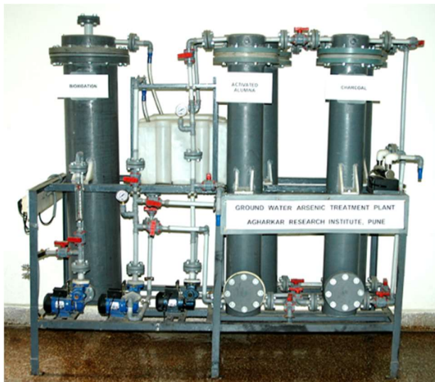
Arsenic Removal Plant
