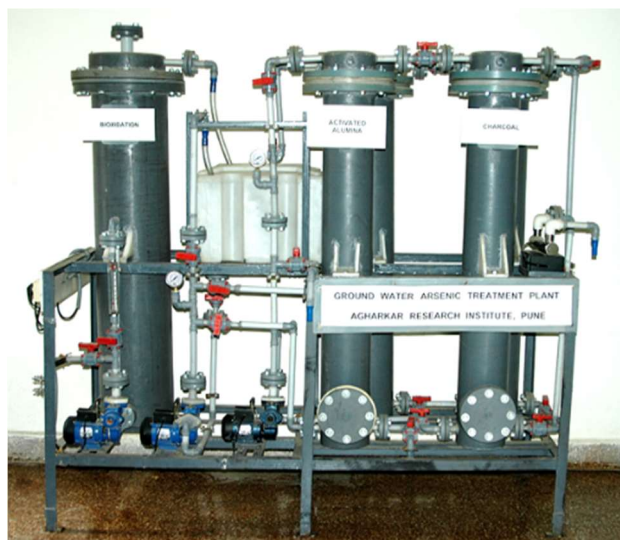
Arsenic Removal Plant
